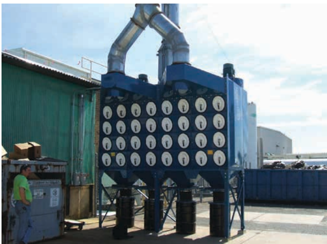
DFO on Thermal Spray 8,500 cfm (14,439 m 3 /h)
