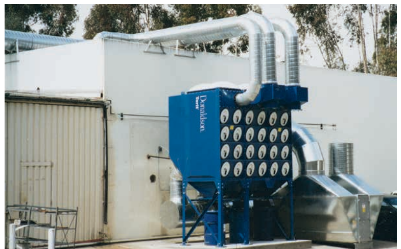
DFO on Metal Grinding 31,000 cfm (52,658 m 3 /h)
