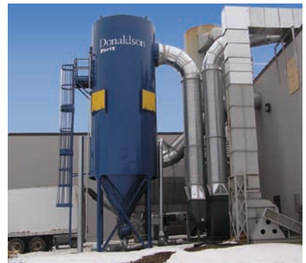
RF - Cabinet Shop 48,500 cfm (82,385 m 3 /h)
