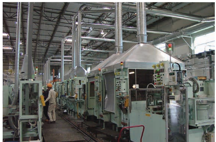
DFO on Welding Fumes 53,000 cfm (90,028 m 3 /h) Left: outside Right: inside
