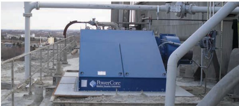
CPV - Multiple Cement Silos 4,800 cfm (8,154 m 3 /h)
