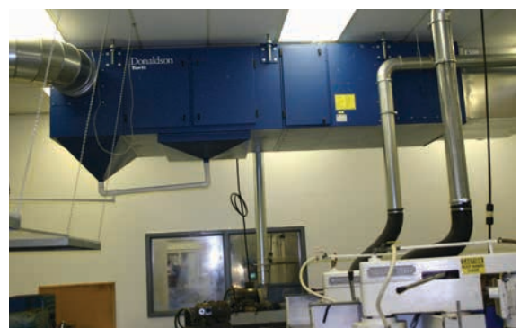
Modular Mediafilter™ on Grinding 2,000 cfm (3,397 m 3 /h)
