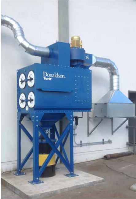
DFE on Rubber Hose Cutting 2,800 cfm (4,757 m 3 /h)
